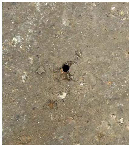
Figure 16: Hole left from DCP testing
