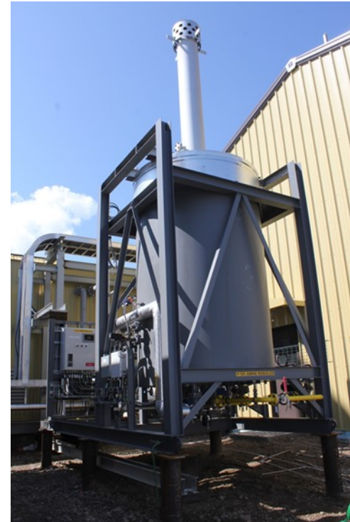
Direct Fired Reboiler
